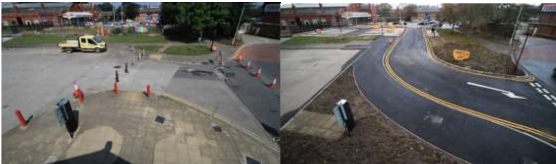
Views of the Bridlington Station plaza work before and after the new exit road was completed.
