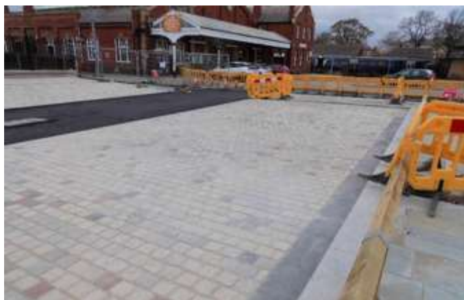
The newly completed disabled and short-stay parking bays at the station plaza.
