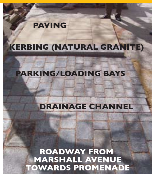
The various surface treatments for Chapel Street laid out for the Town Team at Marshals' depot in Halifax
