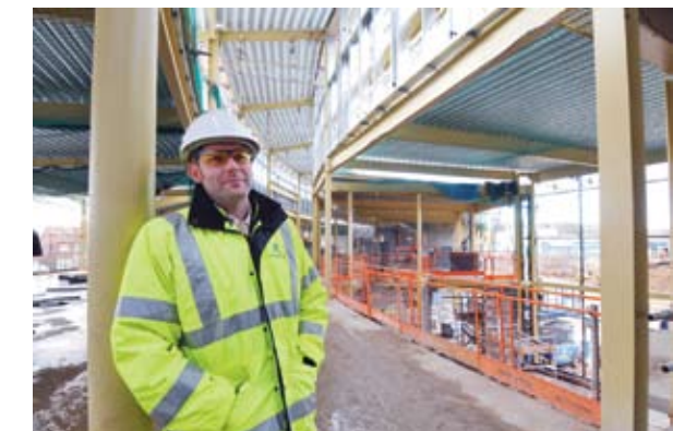
Richard Sellick, East Riding College Project Manager inside the shell of the new building off St. Mary's Walk, Bridlington.
